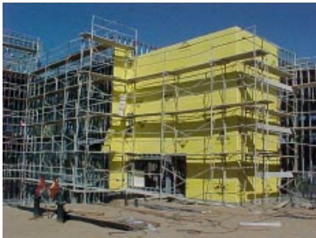
The fiberglass reinforced sheathing installation has begun on the west exterior elevation. This is the first step in the exterior finish application.
