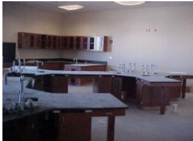
Science Lab covered in drywall dust.
