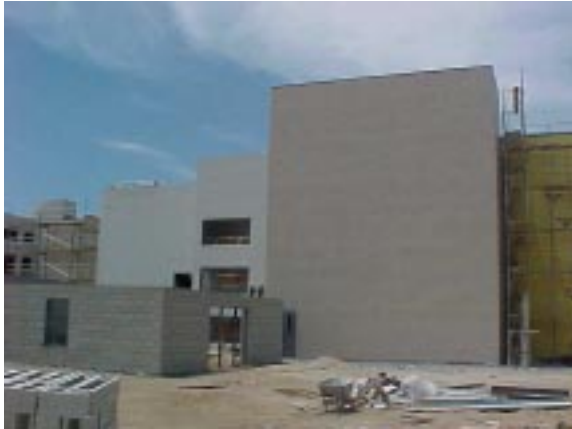
East elevation, stone veneer @ stair tower, EIFS system finish & mech. yard block wall
