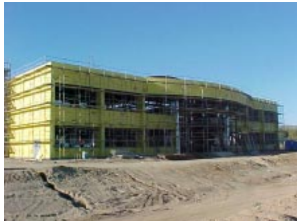
North elevation, fiberglass reinforced sheathing installed, styrofoam installation is the next step in the EIFS System
