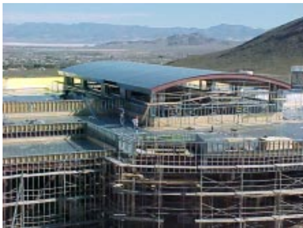
South elevation, roof metal stud framing & welding nearing completion with fiberglass reinforced sheathing continuing.
